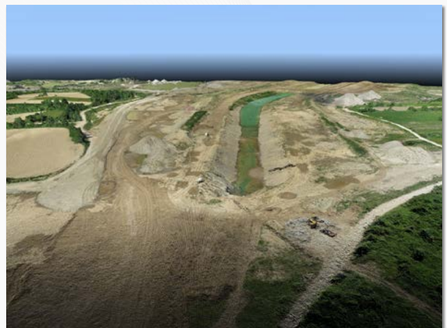
A broader view of the project’s half a billion point 3D cloud.
